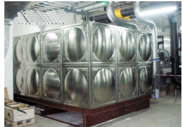
water, chemical or hot water storage
