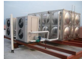
Air conditioning Chilled water storage
